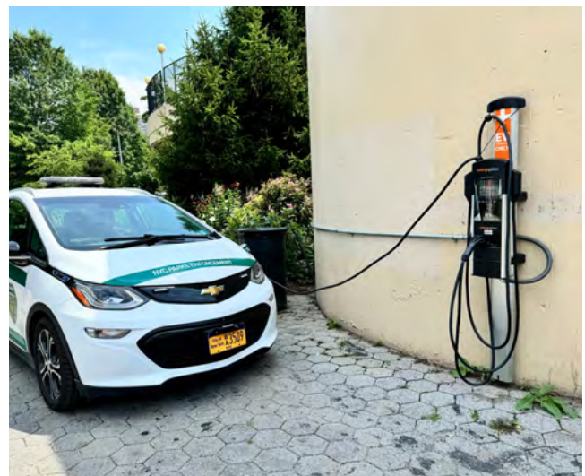
A New York City government-owned electric car charging at Marcus Garvey Park in Harlem, New York City
