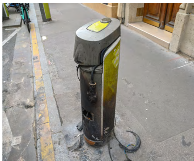
Burnt charging station for electric cars. The charging station was destroyed in the fire. Parking for electric vehicles
